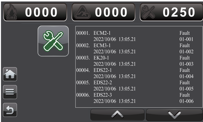
【Figure 2: The Fault events shown on LCD screen.】
